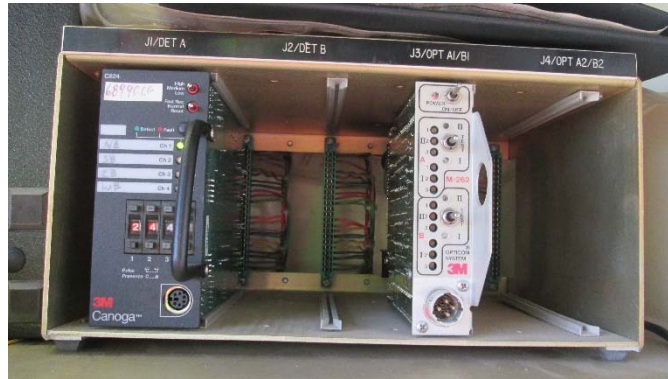
Figure 2 Detection Card Rack at 1st Ave Intersection
