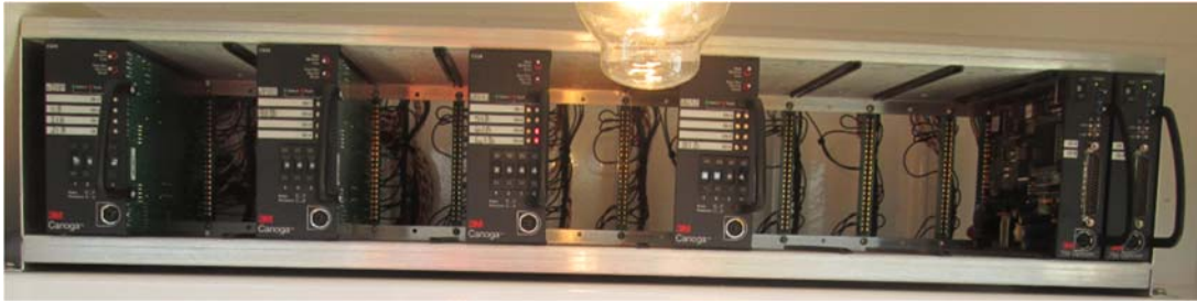
Figure 5 Detection Card Rack at Douglas Road
