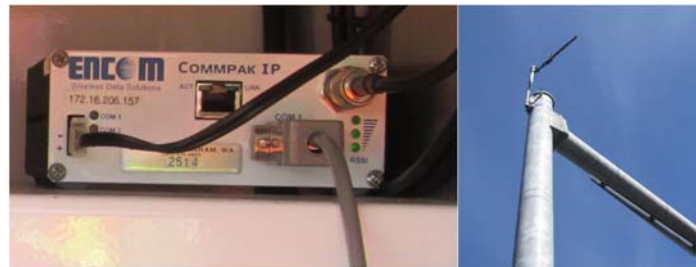
Figure 6 Communication Devices and Antenna Setup
