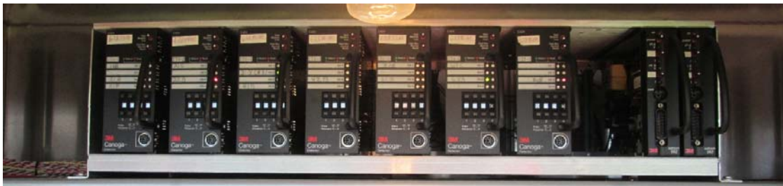
Figure 3 Detection Card Rack at Labounty Drive
