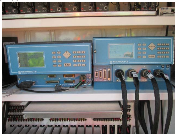
Figure 1 Econolite ASC/2M-1000 Master Controller and ASC/2S 2100 Signal Controller at Retail Driveway intersection
