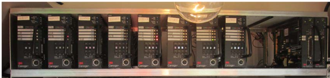
Figure 4 Detection Card Rack at Retail Driveway
